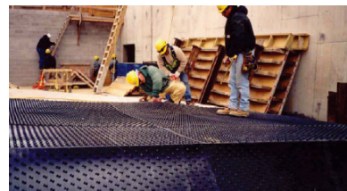
1. Installers attach anchored thermoplastic liners to concrete formwork, then backfill the forms with concrete to lock in the liners.
